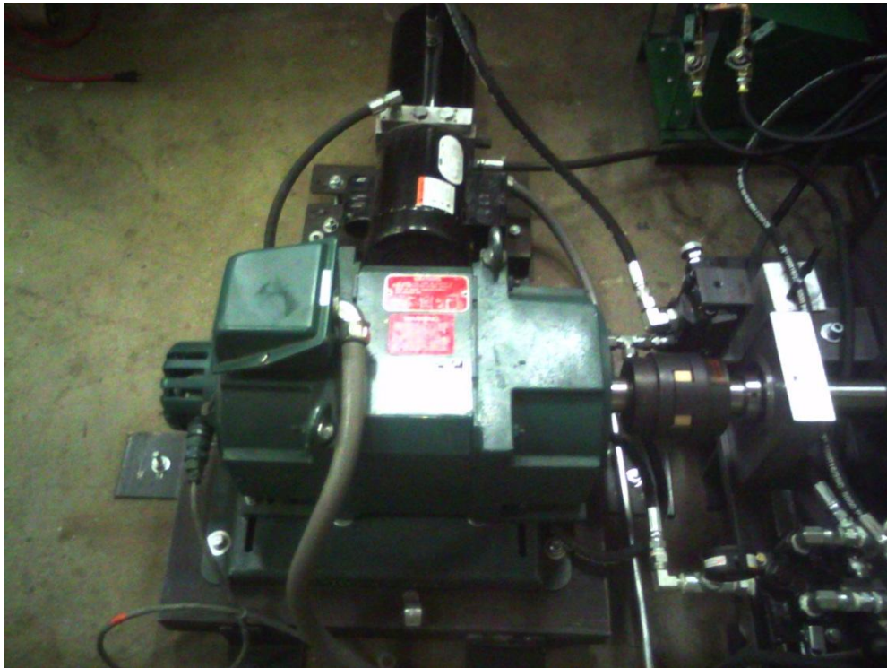
Figure 11 Allen-Bradley 10 hp Motor
